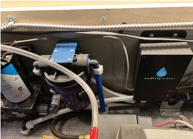
NO Dirty Water (NDW) water filtration
