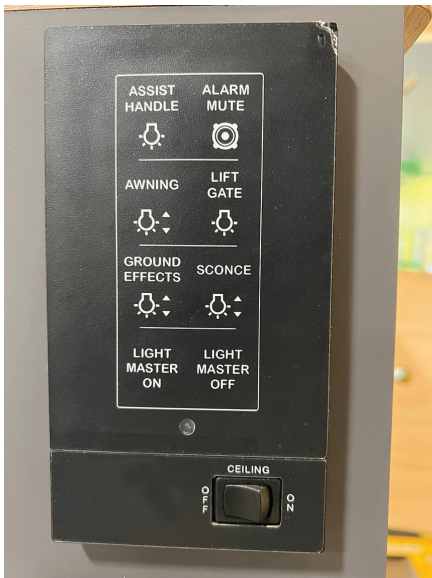
Wireless switch panel, located on entertainment cabinet, at main entrance
