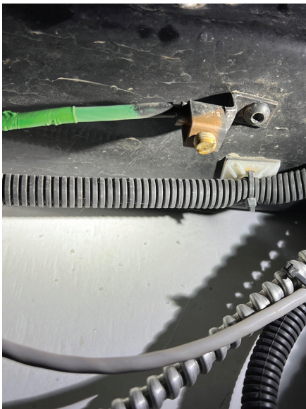
Ground to chassis location
