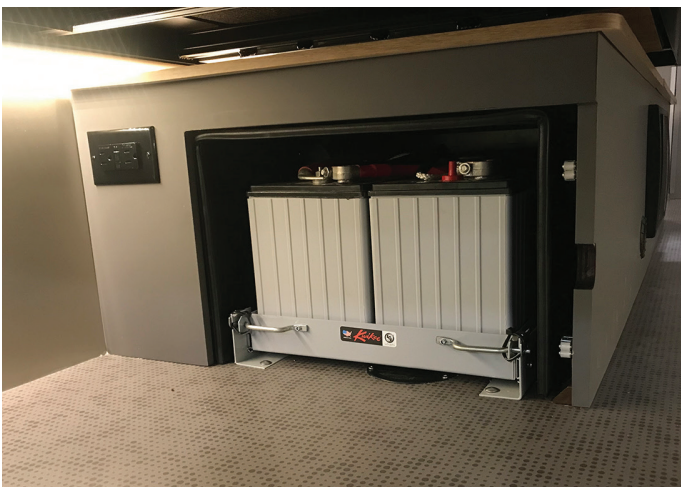
Battery slide-out drawers, locked. Two batteries shown
