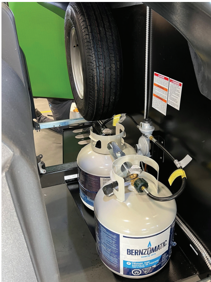
Two propane tanks, secured and connected
