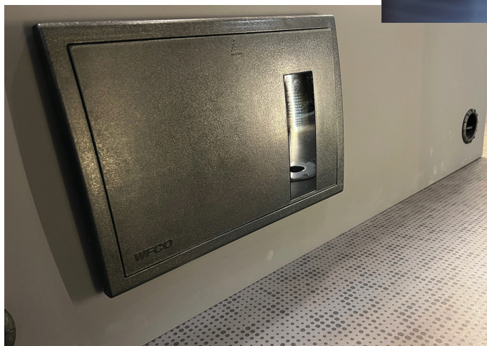
Circuit panel with cover plate closed
