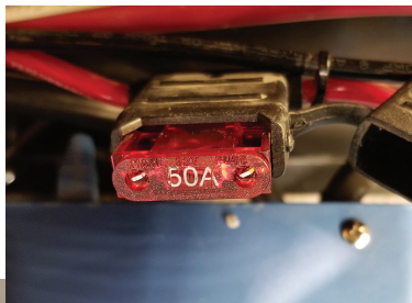
50 Amp in-line fuse, inside utilities equipment cabinet
