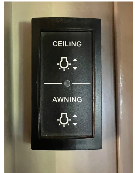
Smaller, 2 button wireless switch panels are located in several locations
