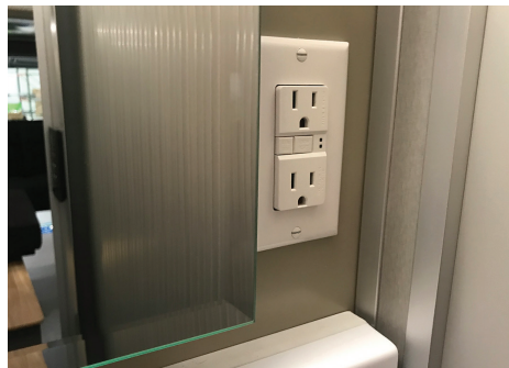
Bathroom AC outlet
