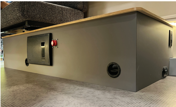
Utilities equipment cabinet, fore
