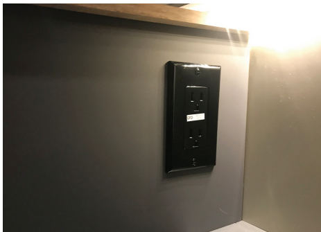
AC outlet on utilities equipment cabinet
