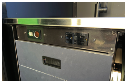
Kitchen power receptacles
