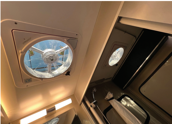
Ventilation fans located over lavatory and kitchen / shower
