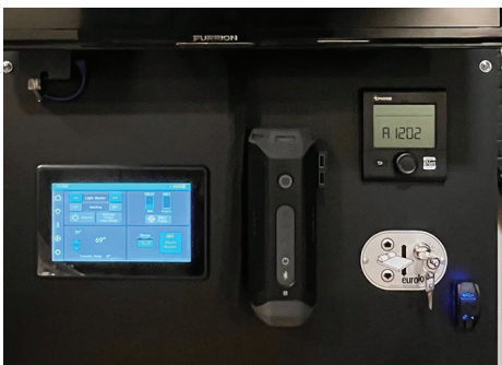
Control system location
