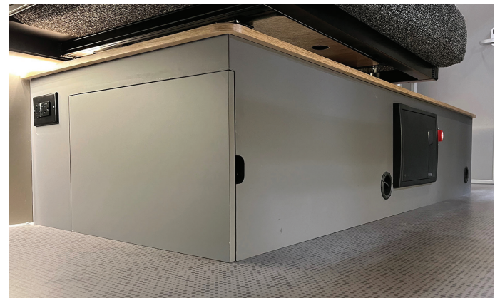
Utilities equipment cabinet, aft
